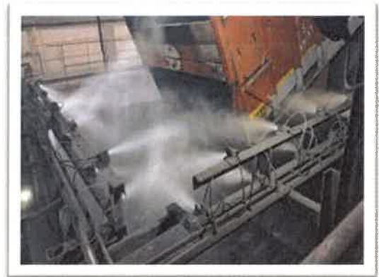
Water sprinkler system
